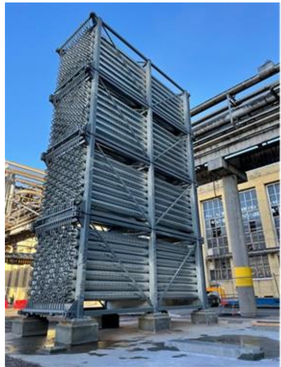
Project partners realizing first installation at Yara International
